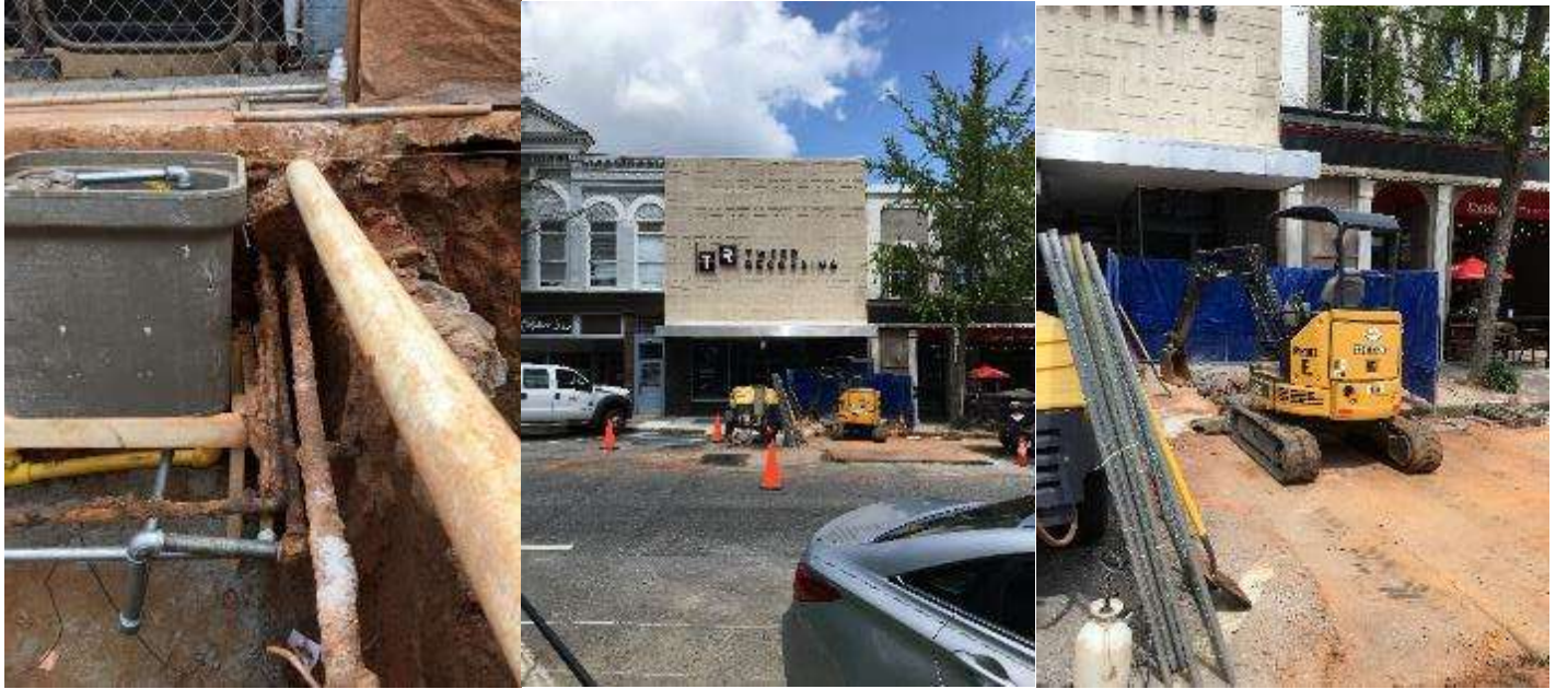
Atlanta Gas light work in removing and replacing corroded pipes. Removing obsolete gas meters and replacing corroded meters.
