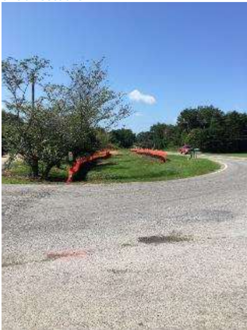
FFT SP#2 East of the Loop on Winterville Rd. Silt Fence and Project Boundaries
